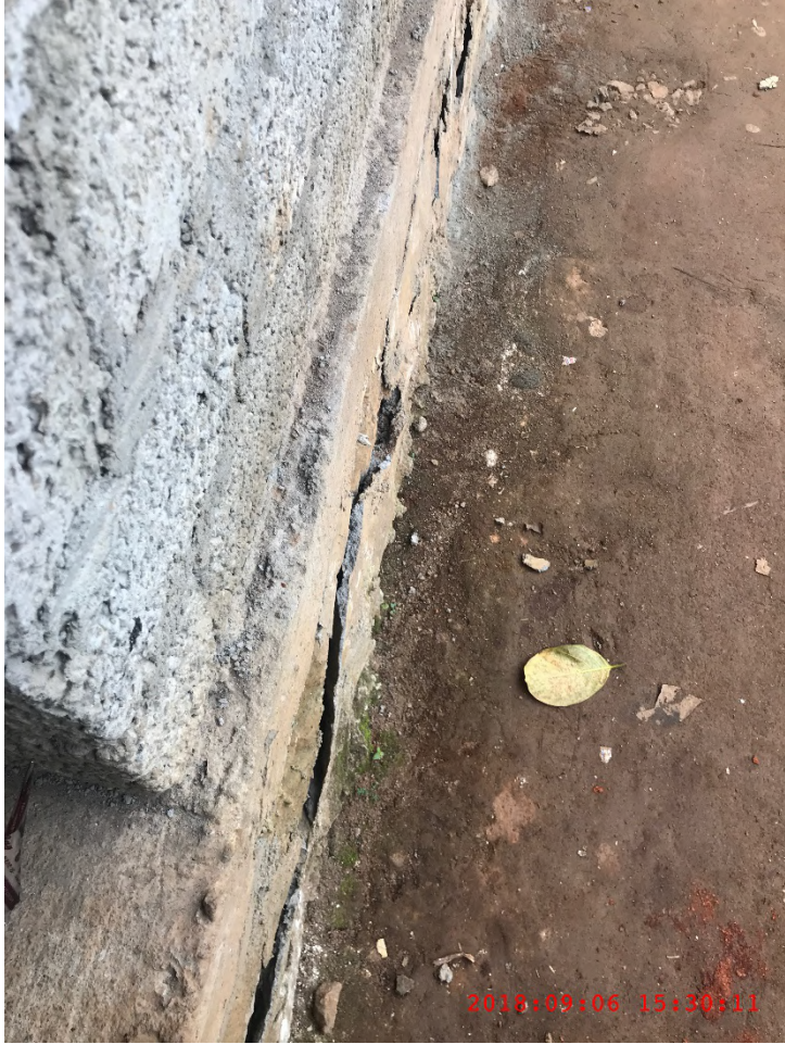
Figure C-2: Another view of the foundation crack @ 9.7918656° N 77.0687362° E
