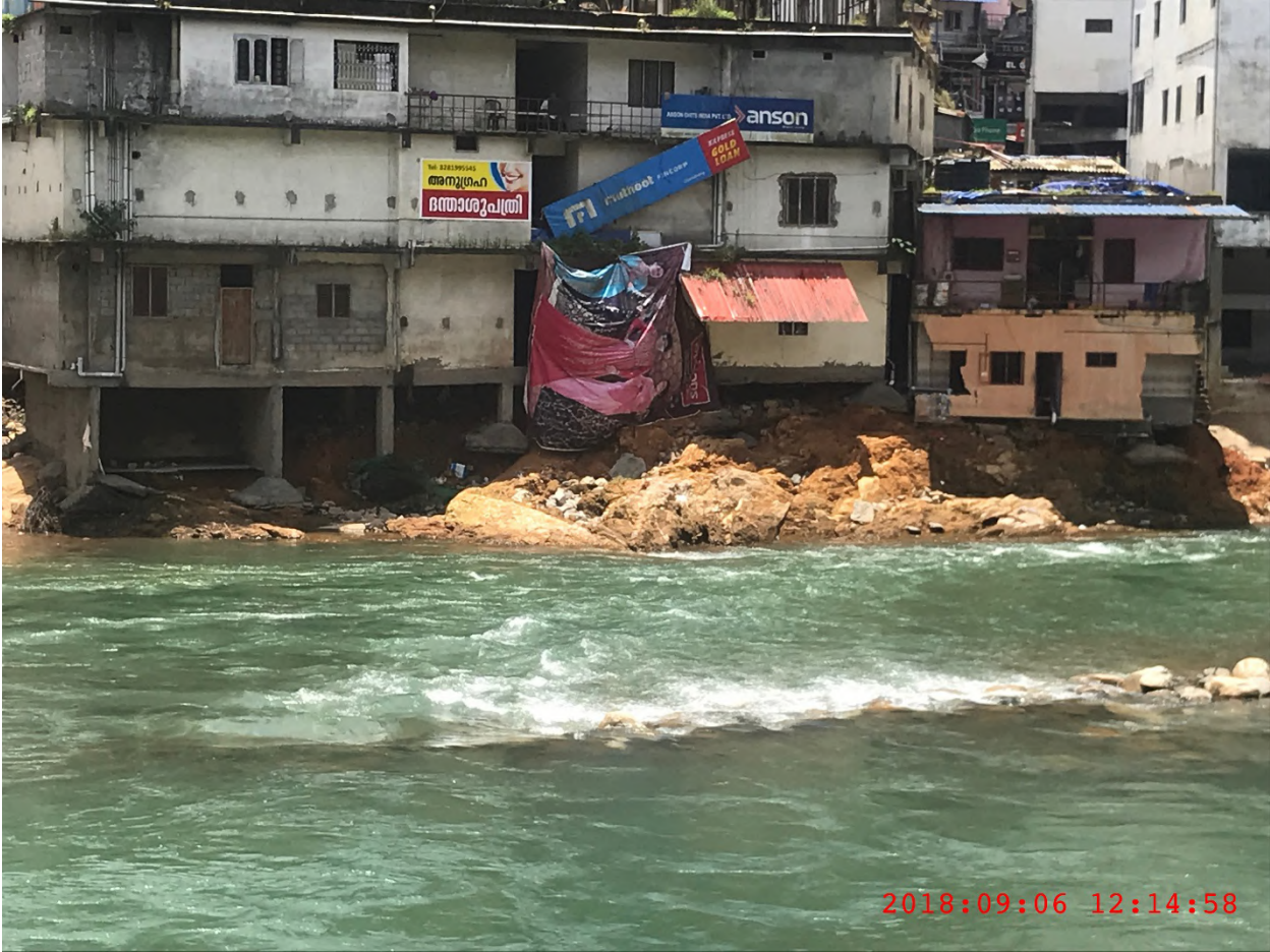
Figure B-1: River erosion @ 9.8575718° N 76.9636035° E
