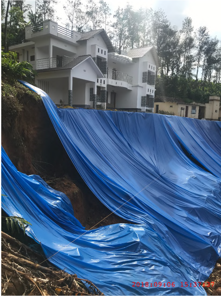
Figure A-11: Large landslide in front of the newly built house @ 9.7925061° N 77.0680952° E
