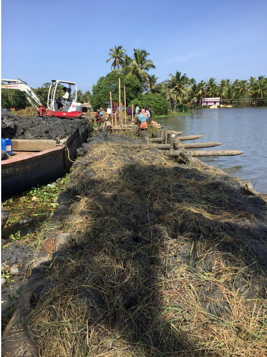
Figure 5.5: A major bund failure of roughly 50m long near Kainakari @ 9.5029947 0 N 76.3749555 0 E. The left side of the bund in the photograph is the lake and the right side of the bund is the flooded fields.
