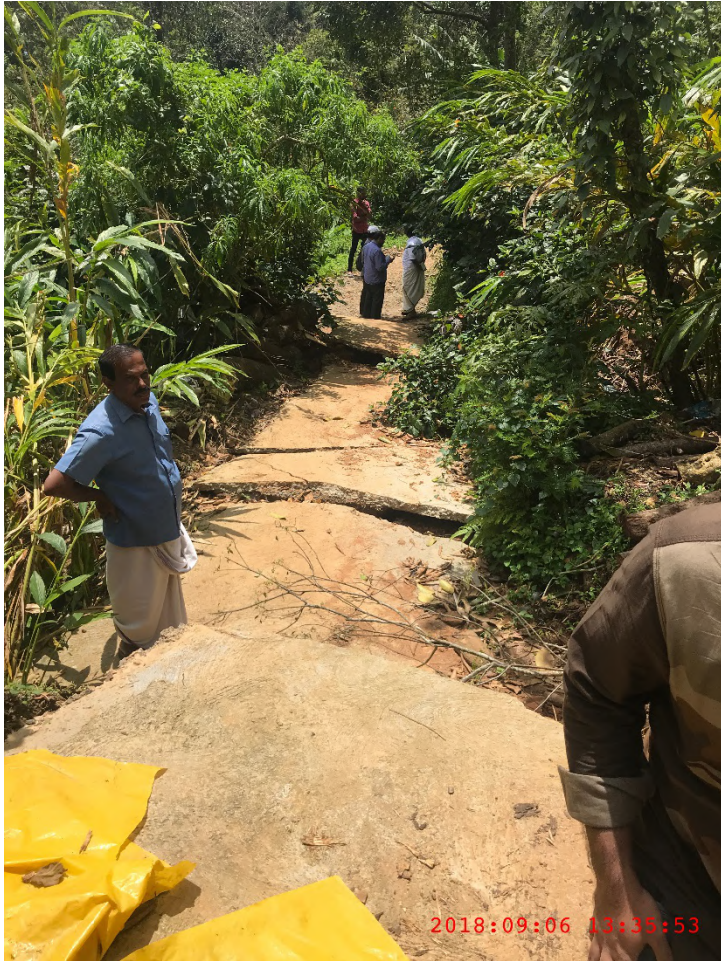
Figure A-8: Driveway to the house destroyed in landslide @ 9.7962622° N 77.0681814° E
