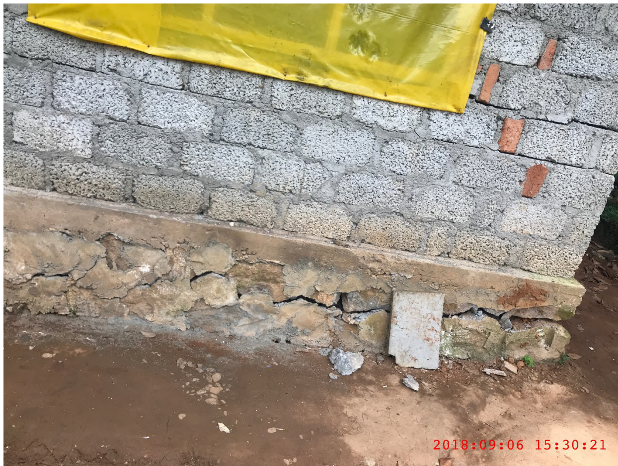
Figure C-1: Foundation of the house cracked due to ground displacement @ 9.7918757° N 77.0687403° E
