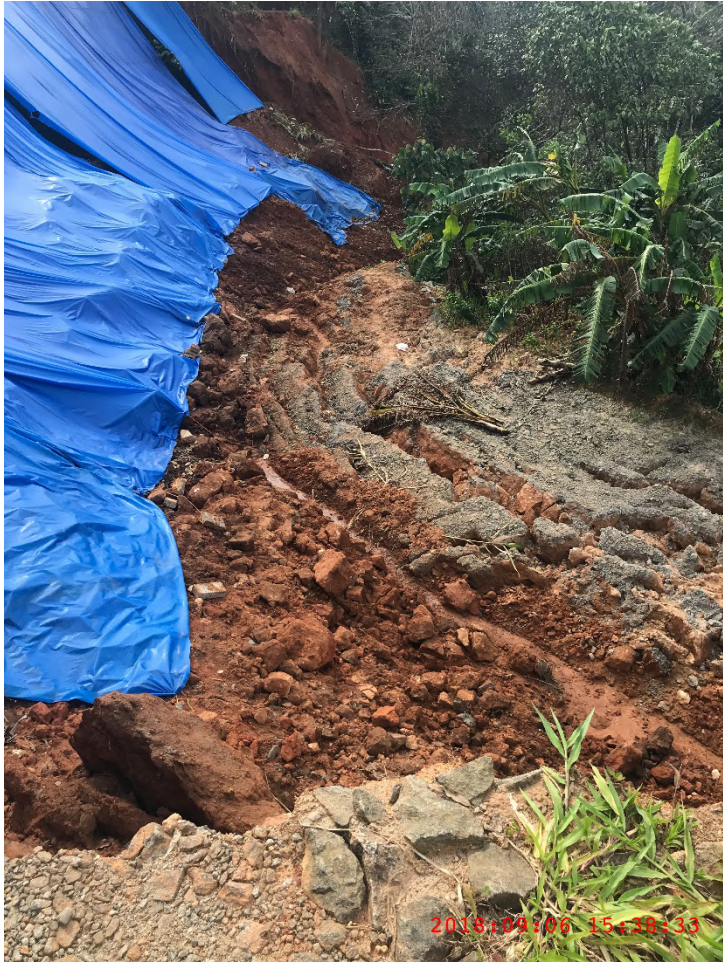
Figure A-12: Head of the landslide @ 9.7925131 o N 77.0680889 o E
