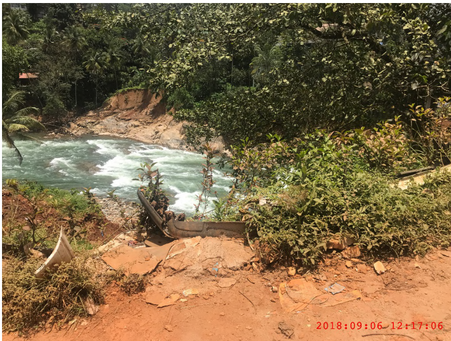
Figure B-3: River erosion @ 9.8585518^{\circ} N 76.9639427^{\circ} E
