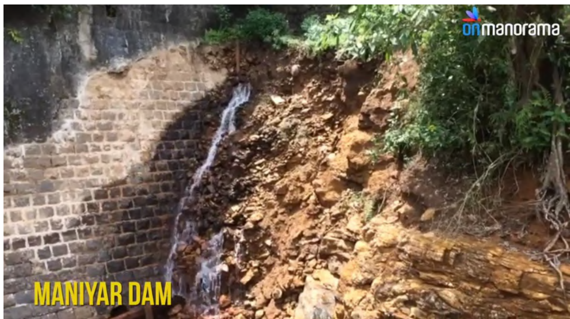
Figure 3.9: Closer view of the slope failure and seepage at the downstream side of the Maniyar dam (Source: manoramaonline.com).
