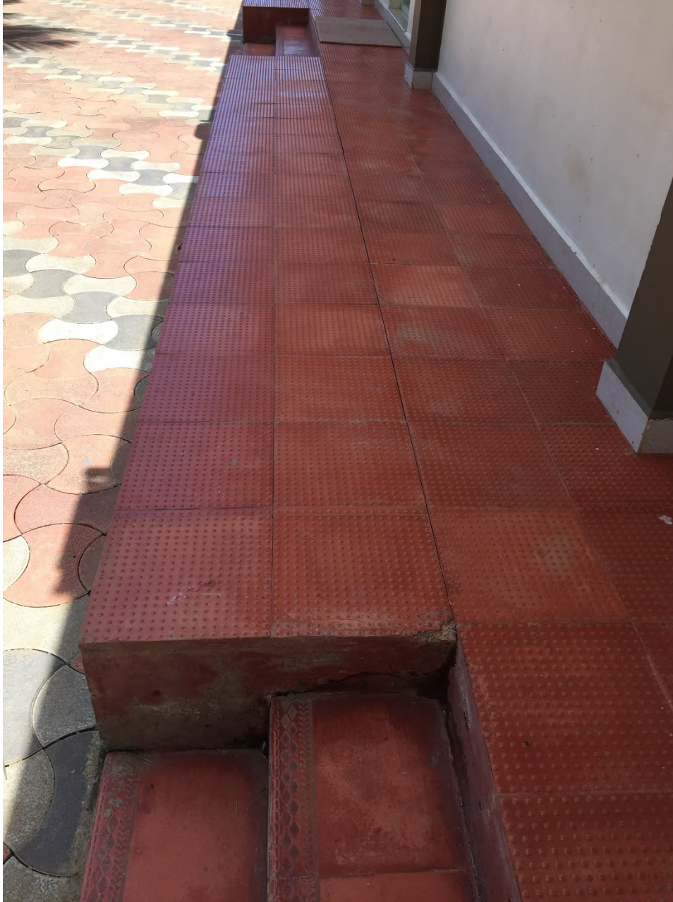
Figure 4.18: Photograph of cracking occurring in the concrete pavers surrounding the pile supported Mar Sleeva Church of Ponga building.
