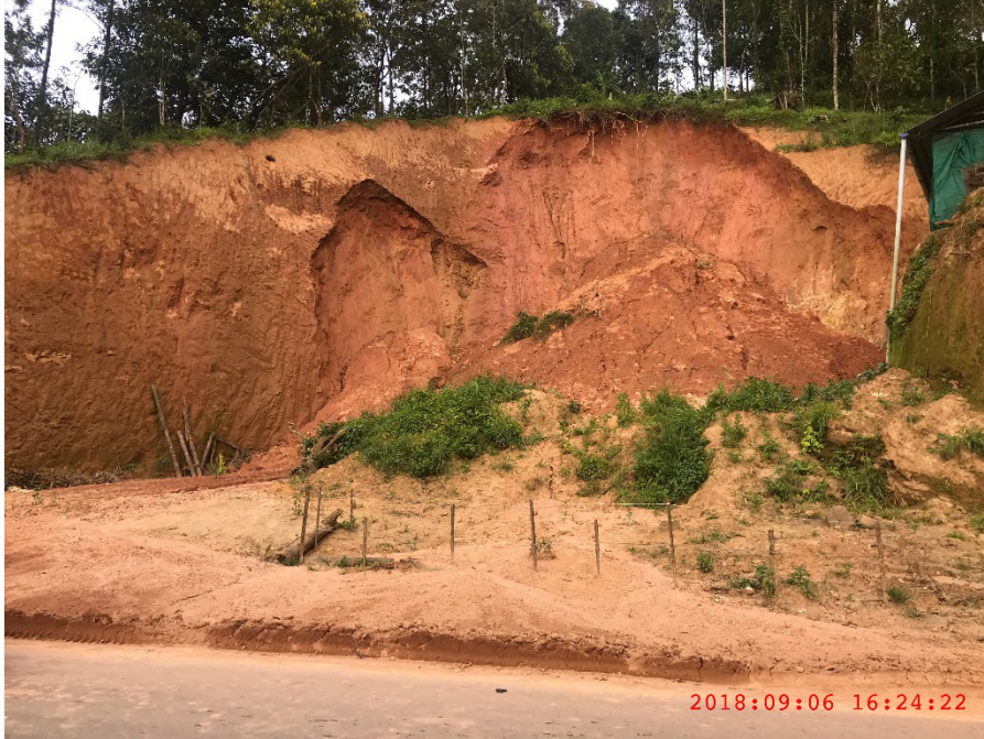
Figure A-13: Minor landslide @ 9.7694732 o N 77.0890198 o E
