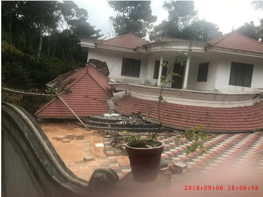
Figure C-4: Building destroyed due to ground movement. An entire floor has been subsided @ 9.8746102° N 77.1193815° E
