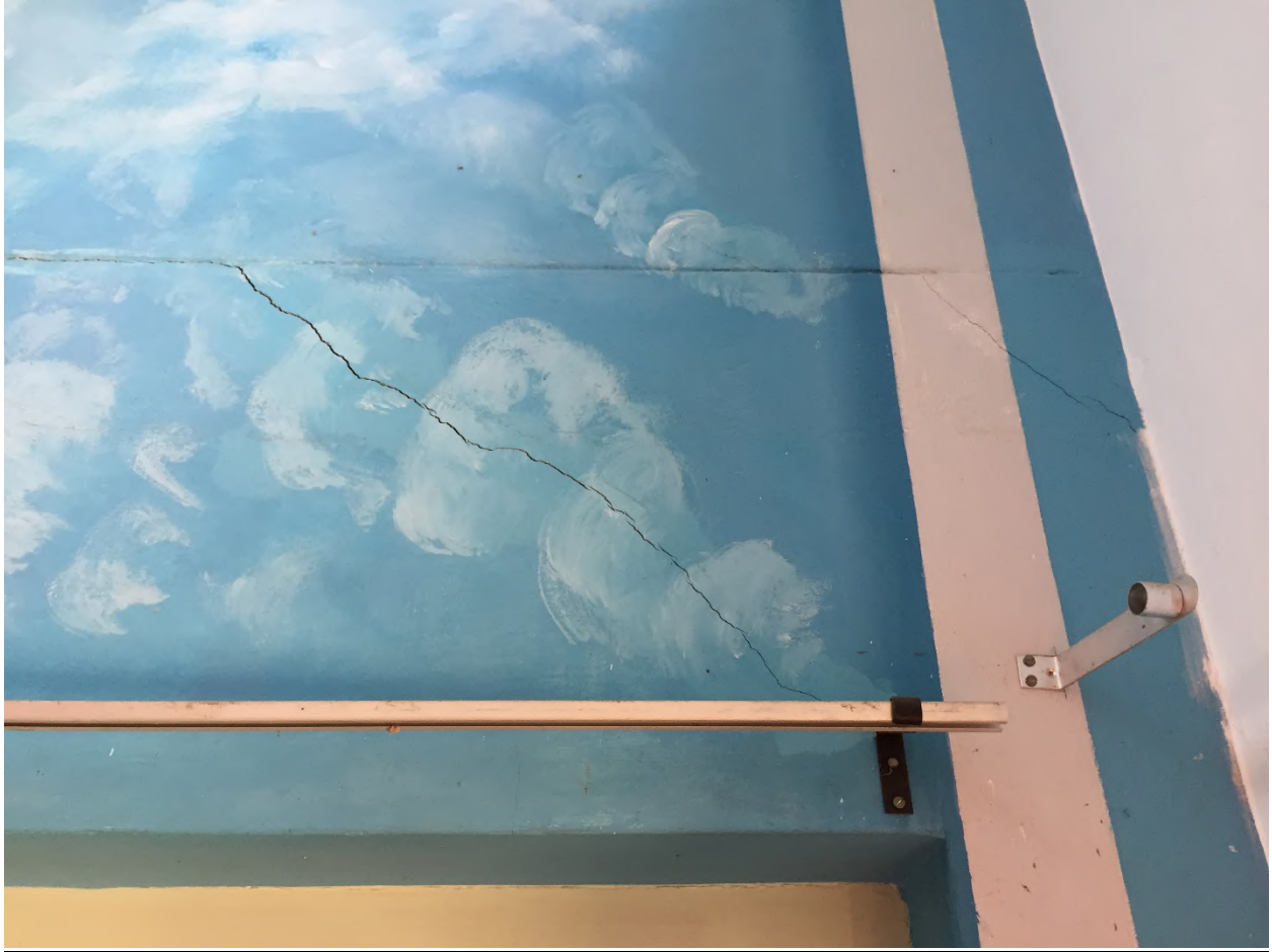
Figure 4.17: Photograph of cracking observed within the back wall of the Mar Sleeva Church or Ponga.
