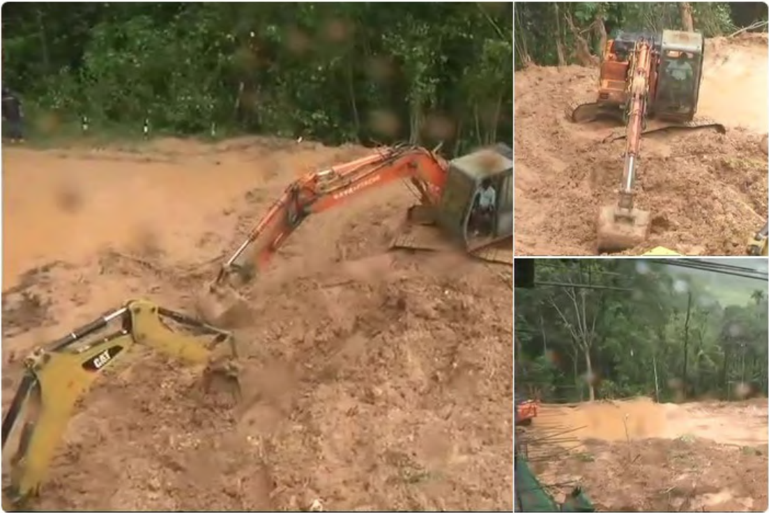
Figure 2.11: Roadway clearing operations at the Kattappana Landslide. The horizontal rebar in the bottom right photograph are also present in many of the photographs taken by the GEER team. Source: Twitter.
