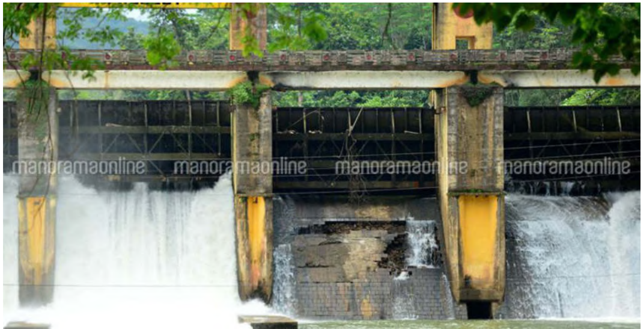
Figure 3.11: Different view of the damage to the downstream surface of shutter-2 at Maniyar Dam (Source: manoramaonline.com).
