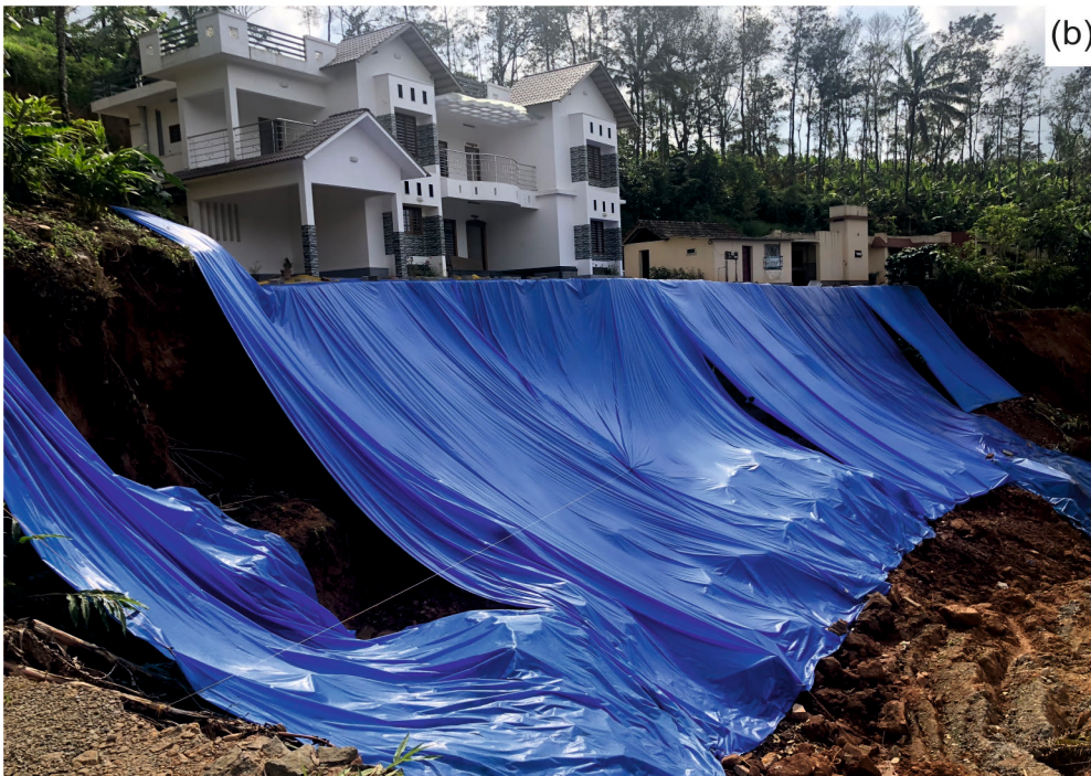
Figure 2.2: (a) Displaced road due to partially failed landslide 9.7968615^{\circ} 77.0675334^{\circ} (b) Cut-slope failure at Nirmala City 9.7925061^{\circ} 77.0680952^{\circ} . Note the modified slope behind the house.
