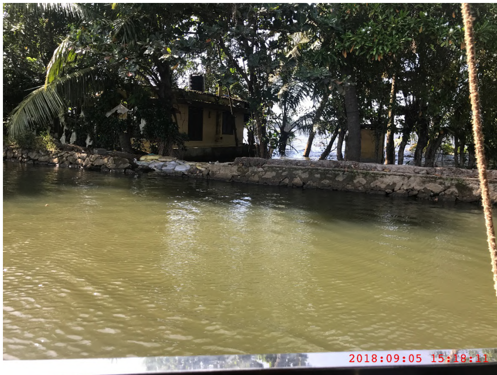
Figure 5.4: A minor bund failure @ 9.5032131 0 N 76.3768638 0 E.
