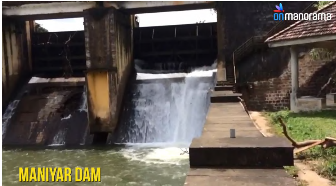
Figure 3.10: Photograph showing one shutter of the dam being closed and the surface concrete blocks been damaged (Source: manoramaonline.com).
