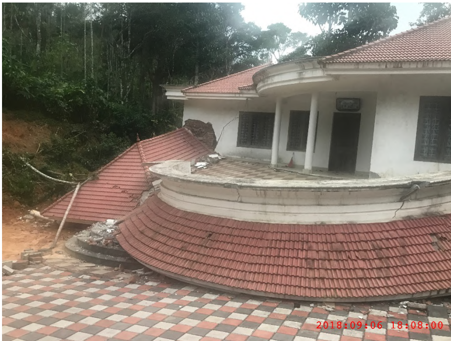
Figure C-5: Building destroyed due to ground movement. An entire floor has been subsided @ 9.8747156° N 77.1193791° E
