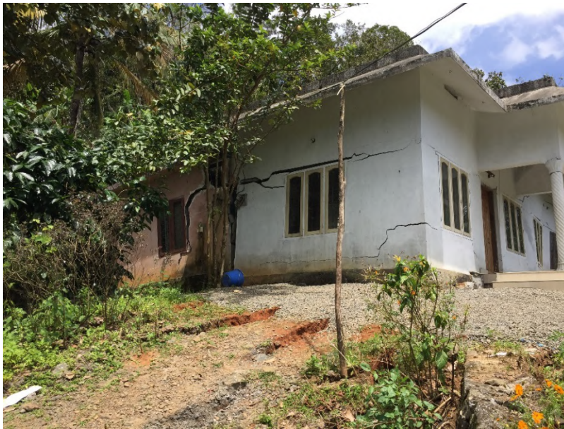
Figure 2.15: Photograph of one of the damaged houses within the Idukki Landslide. Using multiple photographs of this house, this geometry of this house was reconstructed using Photoscan ( 9.7962622^{\circ}\text{N} ; 77.0681814^{\circ}\text{E} ).
