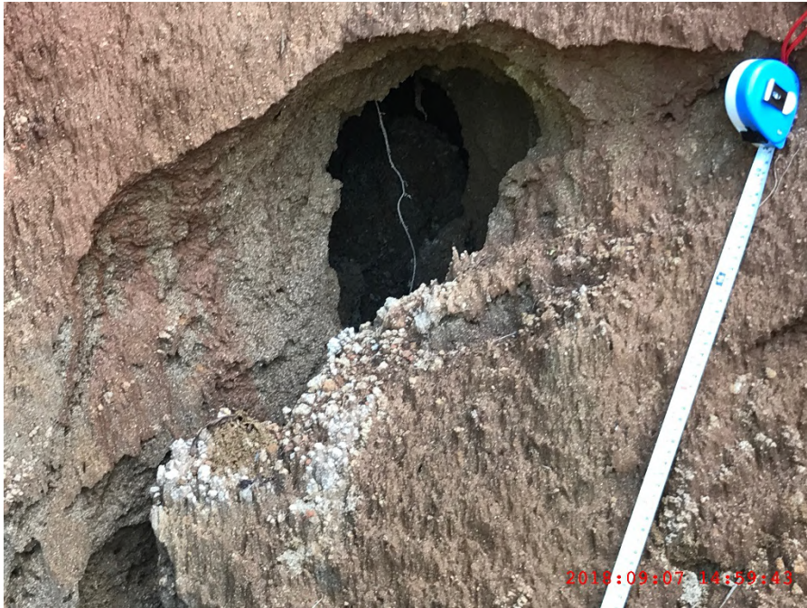
Figure A-20: Example of soil pipping @ 10.0088136^{\circ} N 77.0257626^{\circ} E
