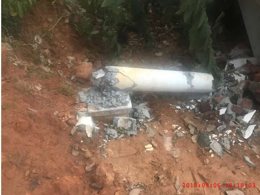
Figure C-6: Column of the building destroyed due to ground movement @ 9.8746397^{\circ} N 77.1193175^{\circ} E
