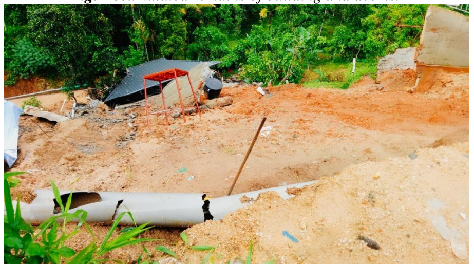
Fig: A view from the crown of the slide depicts the collapsed building.
