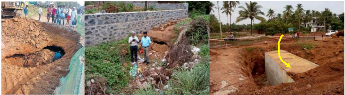
Figure 3.17: Soilpiping incidence occurred in state highway Pallikara, Kasaragod district
