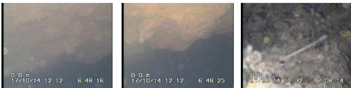
Figure. 4.40 The images taken from inside the pipes (filled with water) by using push Camera
