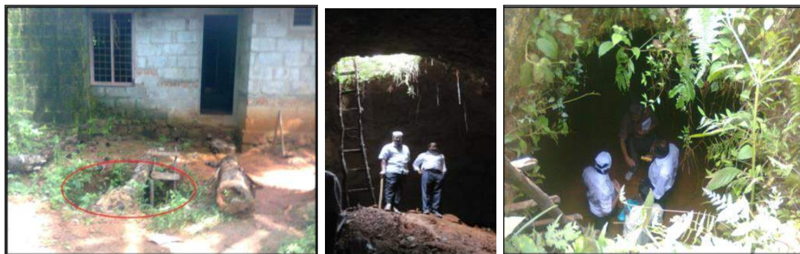
Figure: 7.16 Subsidence occurred in Kollamula village, Pathanamthitta district
