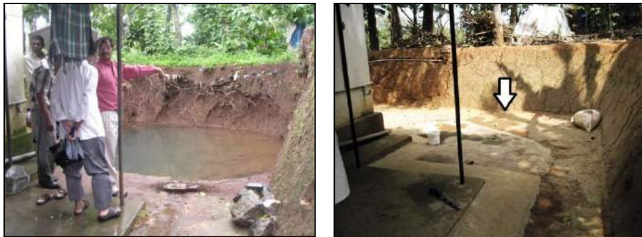
a. Before filling subsided area 2006 b. After filling subsided area 2014
