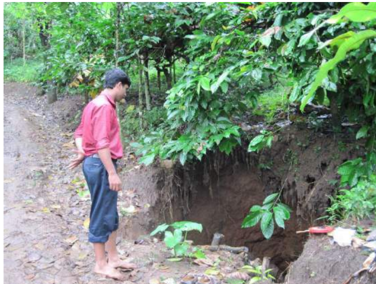
Figure 3.39: A subsidence crater formed along the path way
