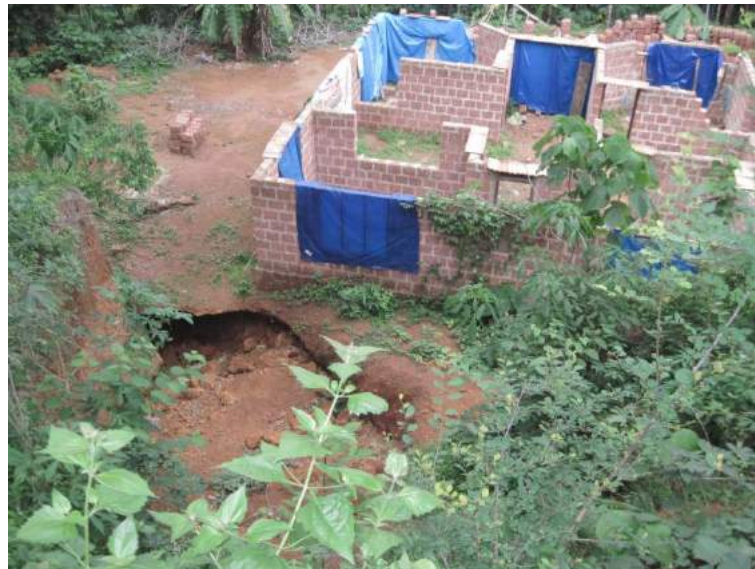
Figure 7.10: Collapsed pipe due to subsurface erosion
