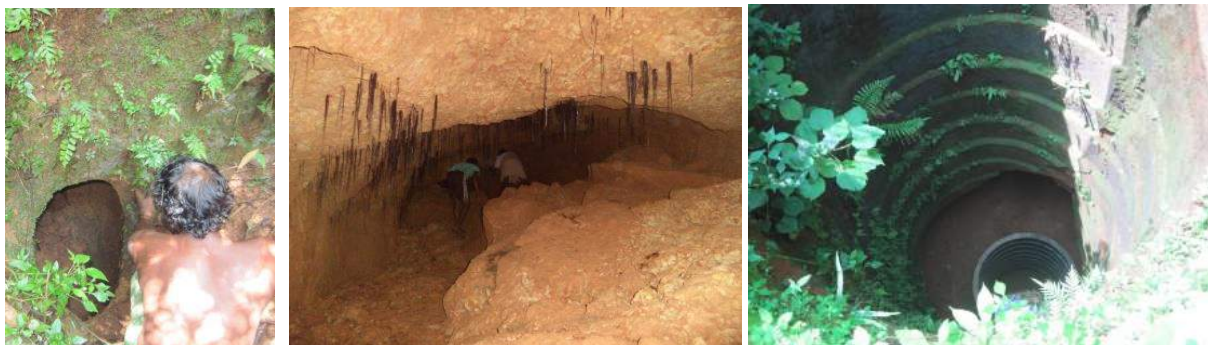
Figure3.15: Piping in Kuttikol, Kasaragod district
