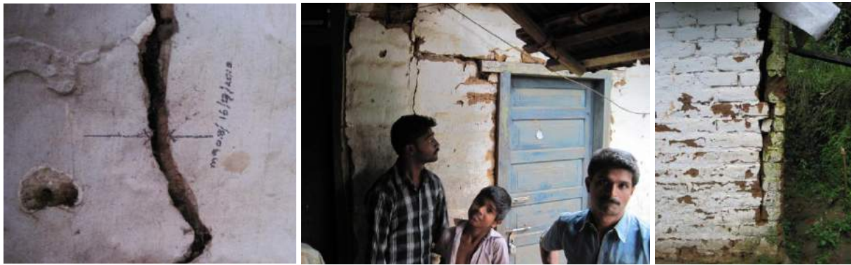
Figure 3.41: Cracks on the wall (Mrs. Jolly's house)
