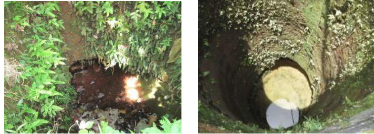
Figure 3.16: Piping and affected well in Erinjilakodu, Kolichal village
