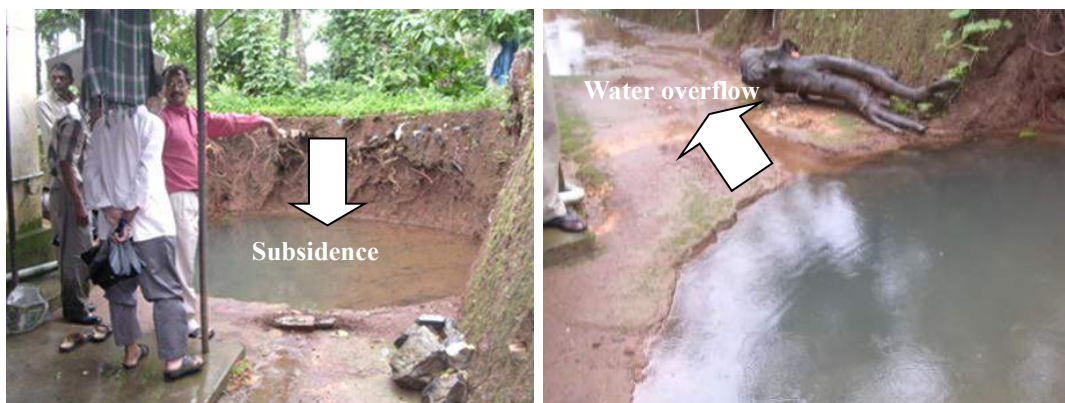
Figure 3.45. Subsidence at Banasurasagar, Vythiri taluk Wayanad district
