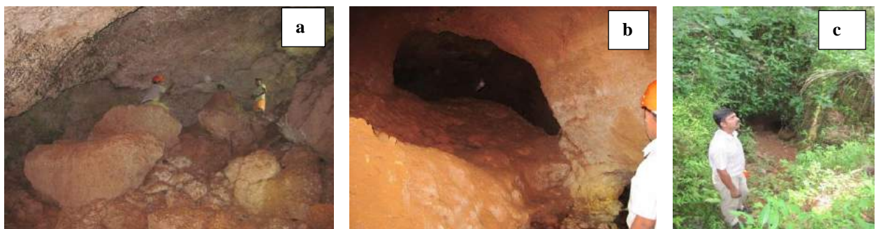
Figure 3.28: Oversized Piping in Lateritic terrain by erosion of clay layer in Vayakkara, Kannur
