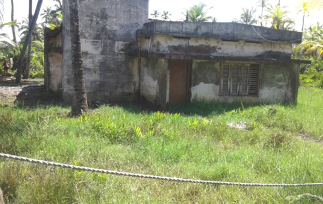
An residential building abandoned after settlement of the floor below the ground.
