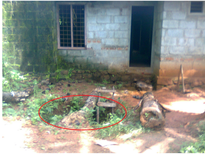
Figure 1: Cavity leading to the soil pipe near the house of Mr. Bhasi
