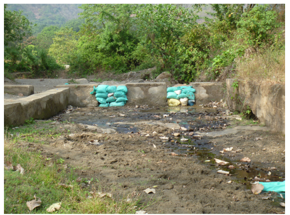
Figure 10: Damaged check dam lower reach of the stream.
