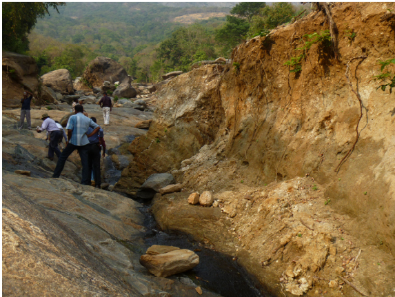
Figure 7: Stream bed and bank erosion. Entire material in the stream bed and 5 meter thick sidewall was also removed.
