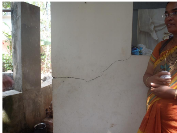
Damage to walls of houses
