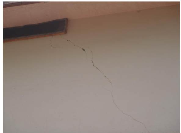
Damage to walls of houses
