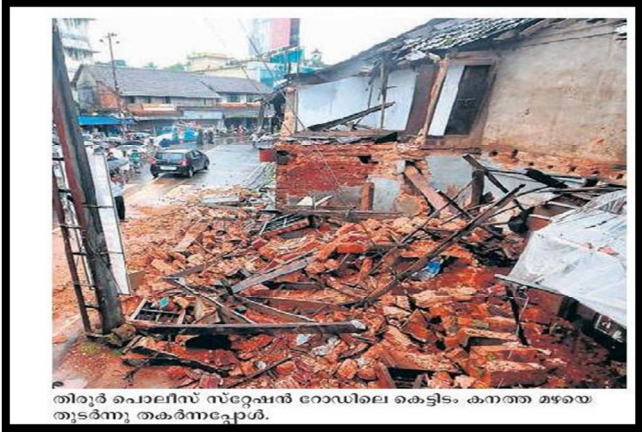
Building collapsed due to heavy rain, Thiroor, Malappuram 03.08.2014
