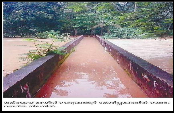
Flooded Bridge at Peringalloor, Kollam 24.08.2014
