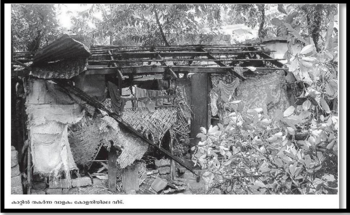
House damaged at Valakam colony Kottarakkara, Kollam 20.06.2014
