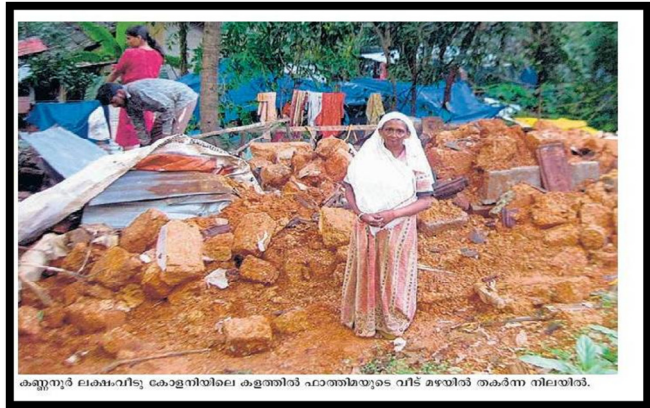
Completely damaged house at Kannannur, Palakkad 03.09.2014
