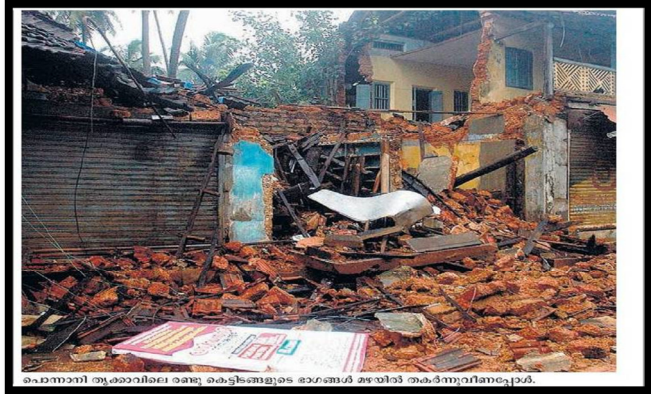
Building collapsed at Ponnani, Malappuram,03.08.2014.
